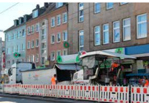
Roadworks in Essen Altendorfer main street Special features: On a route of about 800m, over 80 valves, shafts, hydrants and overhead cables, installation of LOA 5D.
