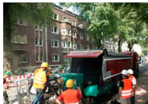
District administration Duisburg Special features:Asphalting in the town centre with many obstacles. Partial discharges and the feeding of footpath pavers.
