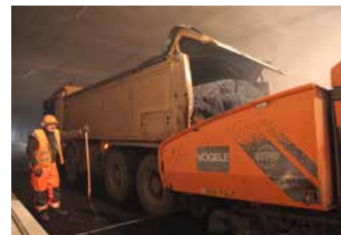
Construction site in Munich Luise-Kisselbachstr. Special features: Deployment in tunnels with temperature-reduced asphalt.
